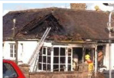
The damaged roof caused by fire at the Coast Road property
