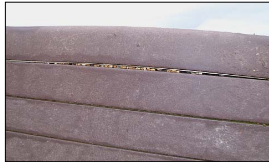
Deformation caused by sediment ingress
