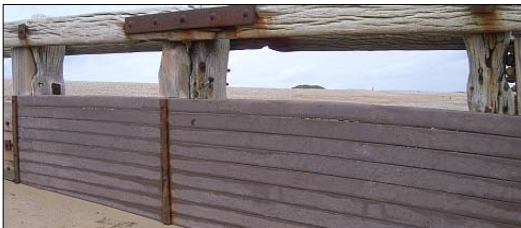
The plastic panel on groyne GC16
