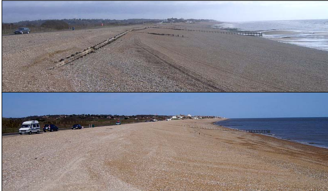
Post storm recovery and repair at Herbrand Walk flagpole Top: Exposed Wavescreen near the flagpole at end of March Bottom: Reprofiled beach on 15 th April 2010
