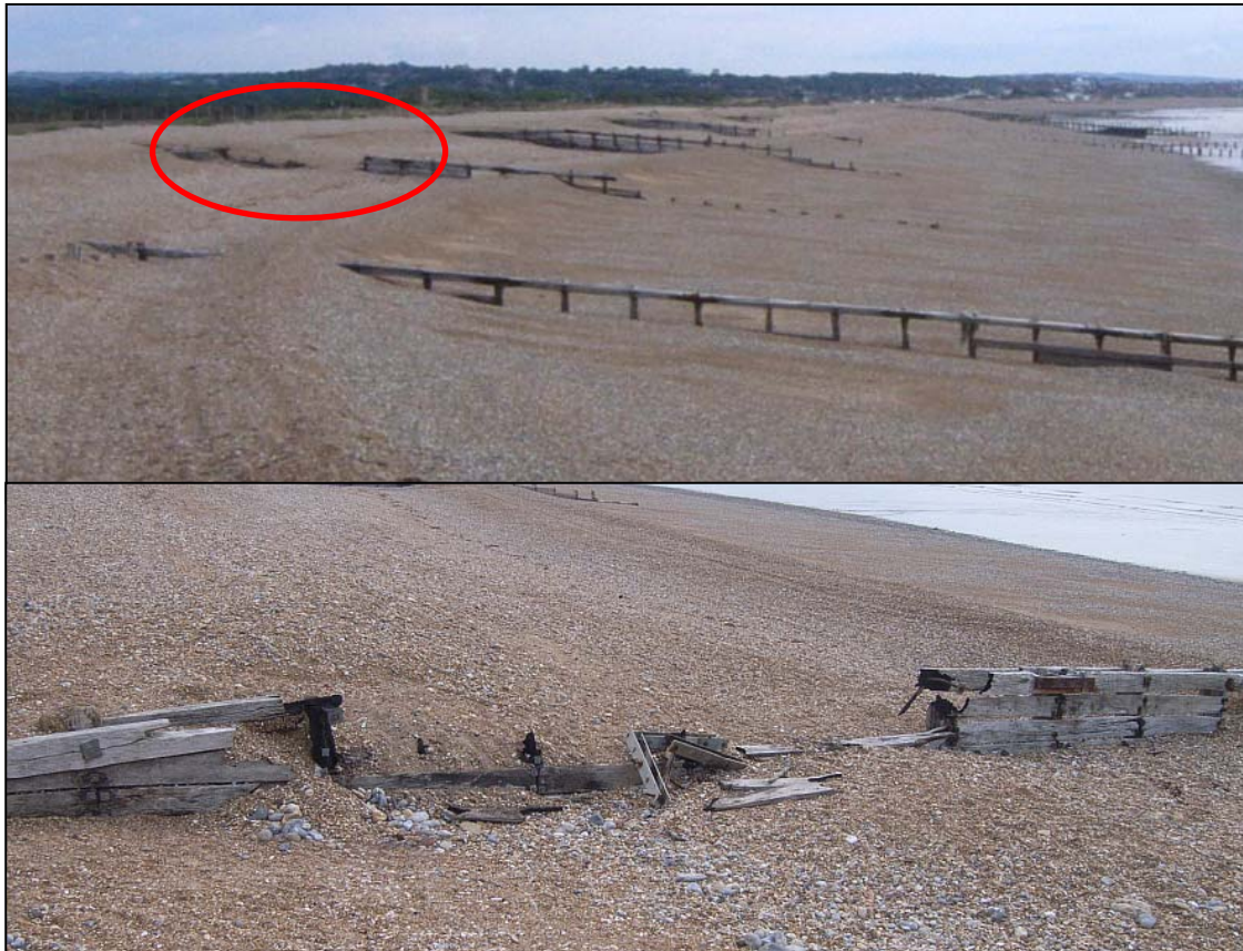
Top: Fire damage to groyne GC03 (circled) Bottom: Detail of affected area.
